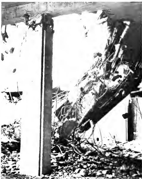
Photo 6. Flexural damage in column of San Fernando Road overhead [2].
